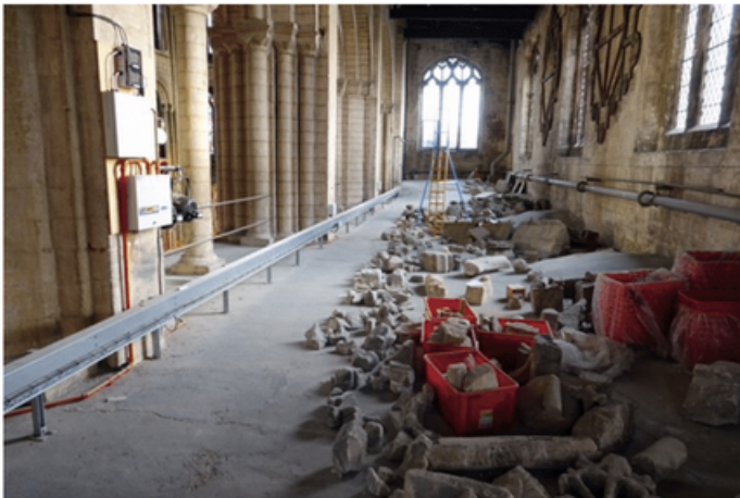
Trip hazards on the Triforium level: Raised cable conduit to the left and archaeological rubble to the right.
