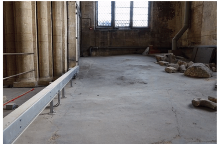
Example of uneven floor of Triforium level.
