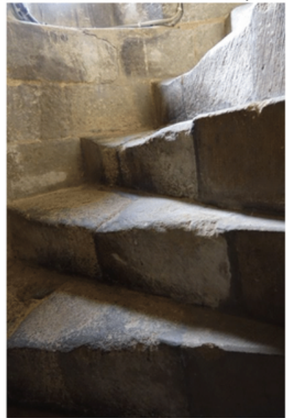
Example of uneven step.
